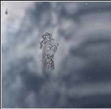
Bat Droppings Stains
